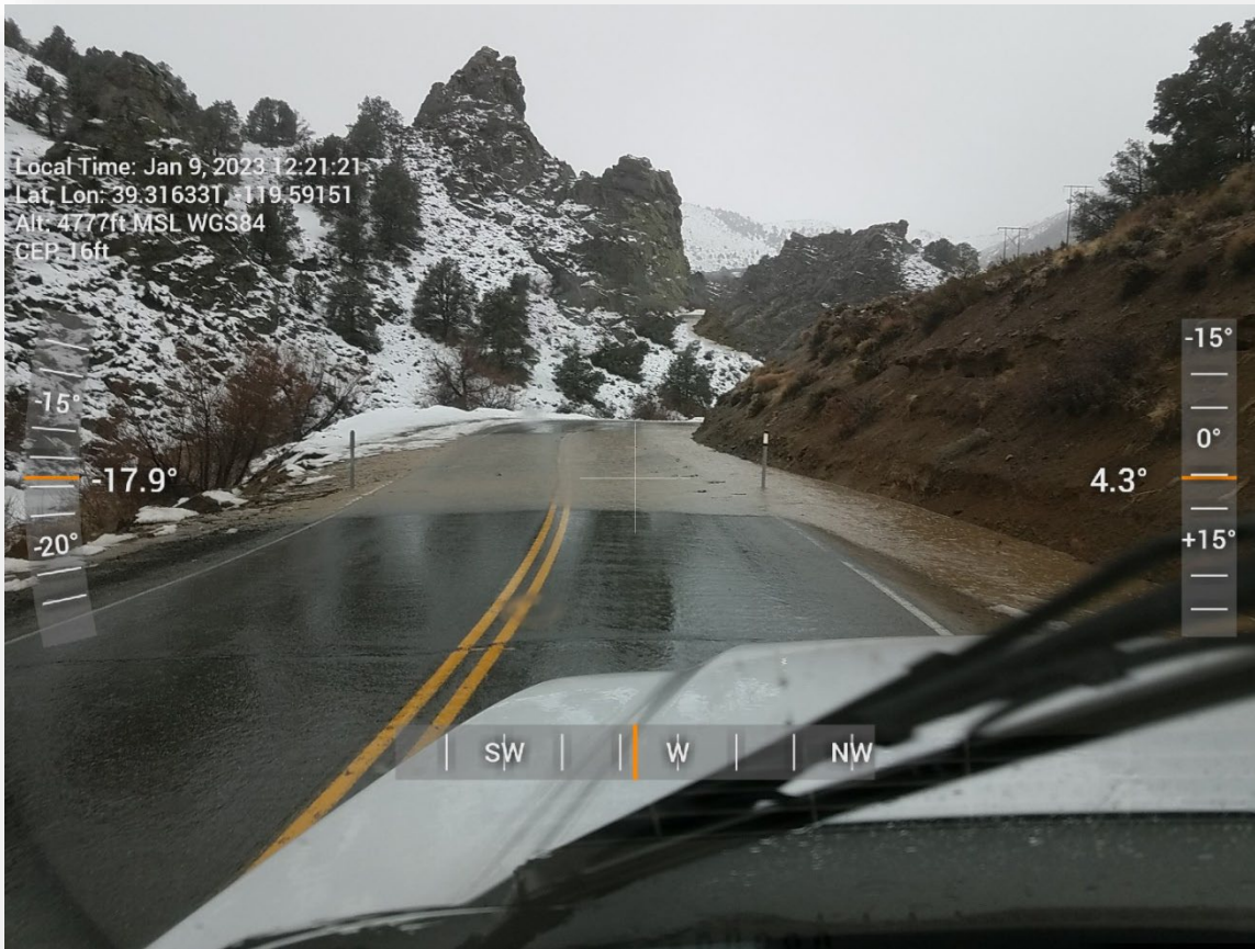
Roadside channels become filled with sediment and overtop, causing sheet flow across the roadway.
